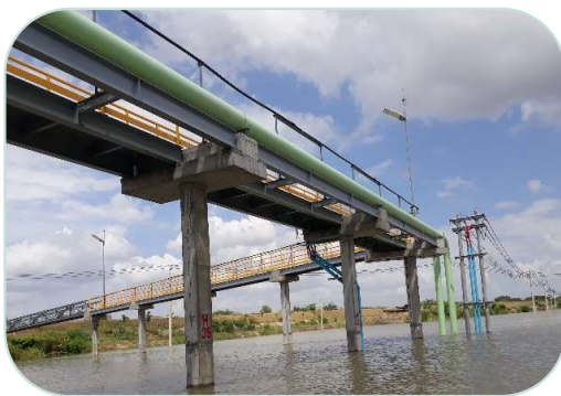
Water Pipeline (Intake & Discharge)
