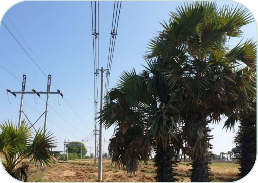
6.6kV Overhead Transmission Line
