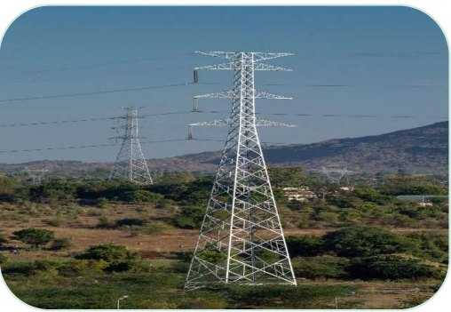
230 kV Transmission Tower
